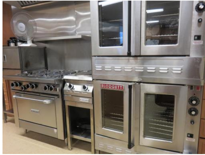
A smaller, more user-friendly gas stove, an electric hotplate and two large ovens replace the former gas and electric stoves.
