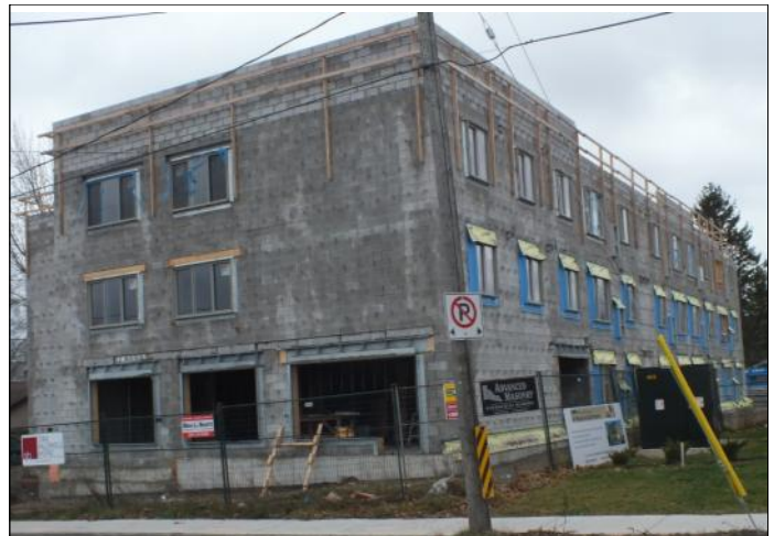
The MennoHomes affordable housing building is going up beside the Woolwich Community Services building on Church Street East. A small group of anonymous donors has launched a Matching Funds Initiative for MennoHomes with the goal of raising $500,000 before the end of 2016. New donations in support of this housing project will be matched by the group.
