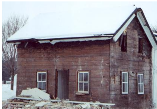
Howard Reist's house was torn down in December, 2004, to provide more room for our new church.
